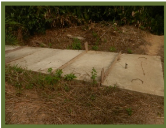
Damage to the Bible School septic system repaired after a stray cow cracked the cement and fell in
